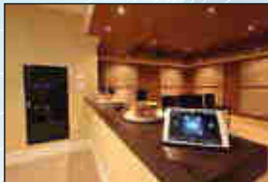
Lighting Automation System
