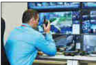
Video Monitoring System (VMS)
