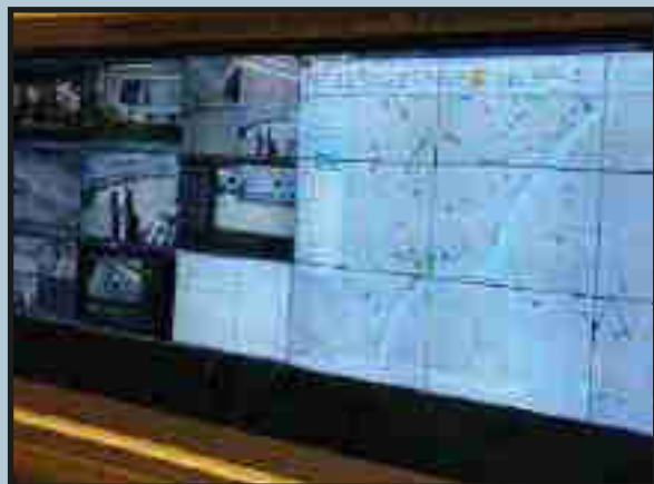
Lafarge Control Room Design
