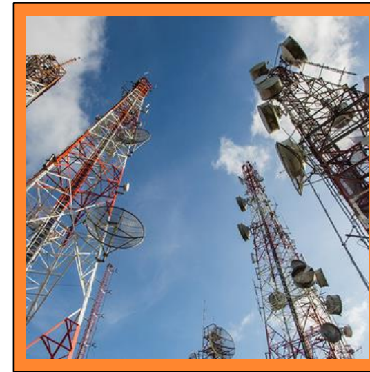
Active & Passive Infrastructure
