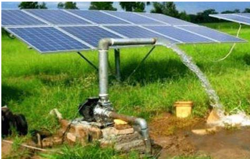
Solar Irrigation Pump
