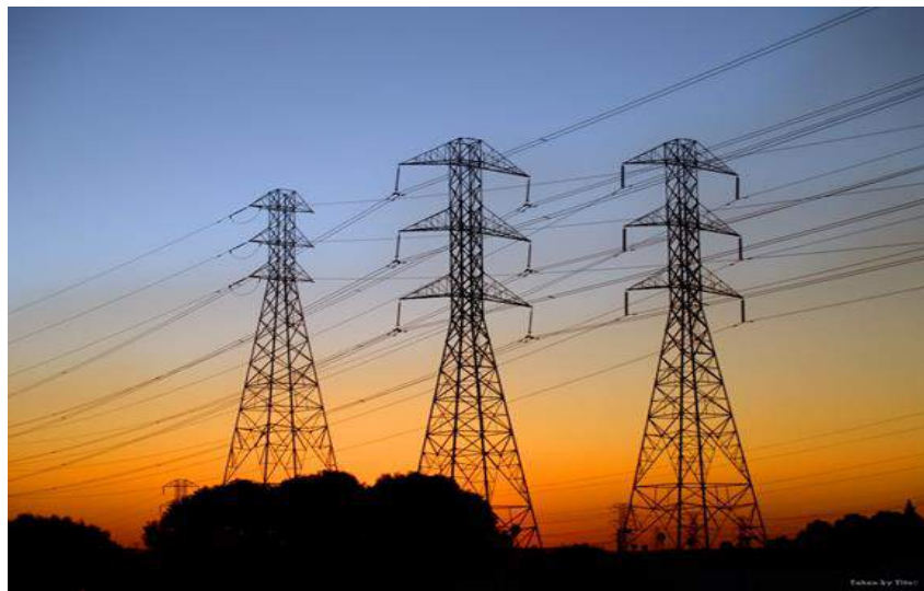
Electrical Transmission Line (Power Evacuation)
